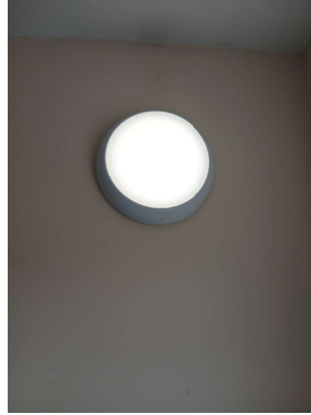
Lighting (Standard and Emergency Lights)
